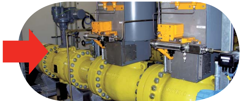
HIPPS prevent over-pressurization by shutting down the source of the high pressure.
