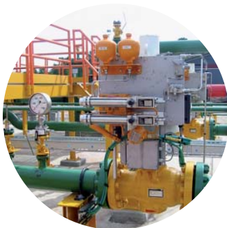
HIPPS with two Mokveld pressure switches protecting Shell Tutong metering station in Brunei.
